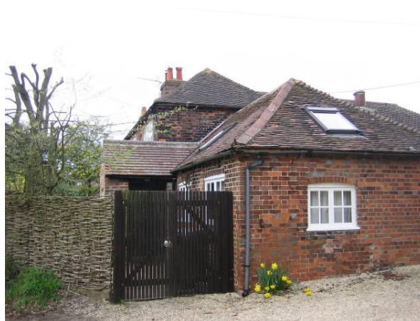
Figure 61: The Old Forge, Hailey Lane. The rooflights sit proud of the roof and detract from the character of the building.
