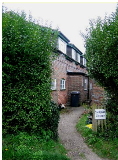
Figure 59: Mell Green Cottages have suffered from inappropriate alterations; in particular, large, mono-pitched dormers.
