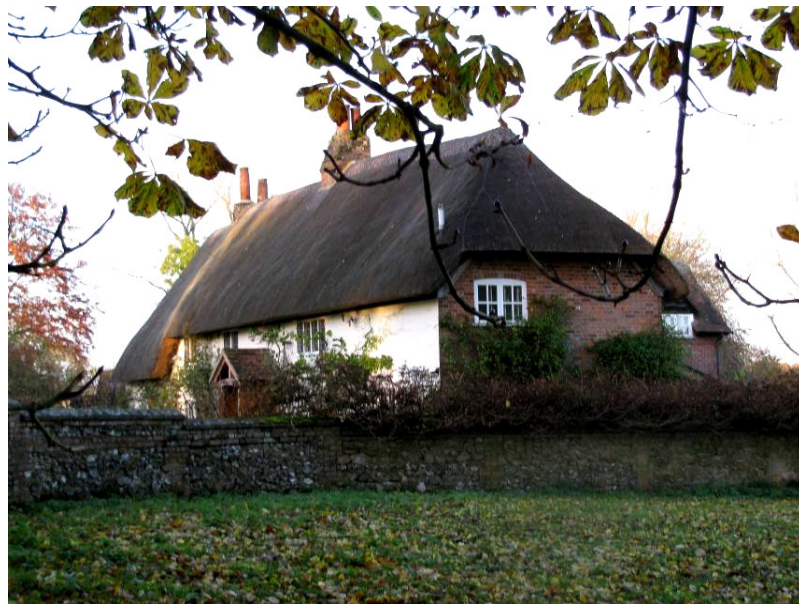
Figure 21: Paxmere House (Grade II listed). The flush ridge has been restrained using liggers.
