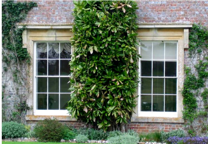
Figure 27: Stone dressed windows with cornices on console brackets at The Old Rectory (Grade II listed)
