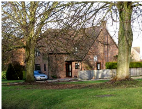
Figure 53: The stained and/or varnished dark brown timber door and window joinery is a non-traditional treatment that fails to reflect the local vernacular.
